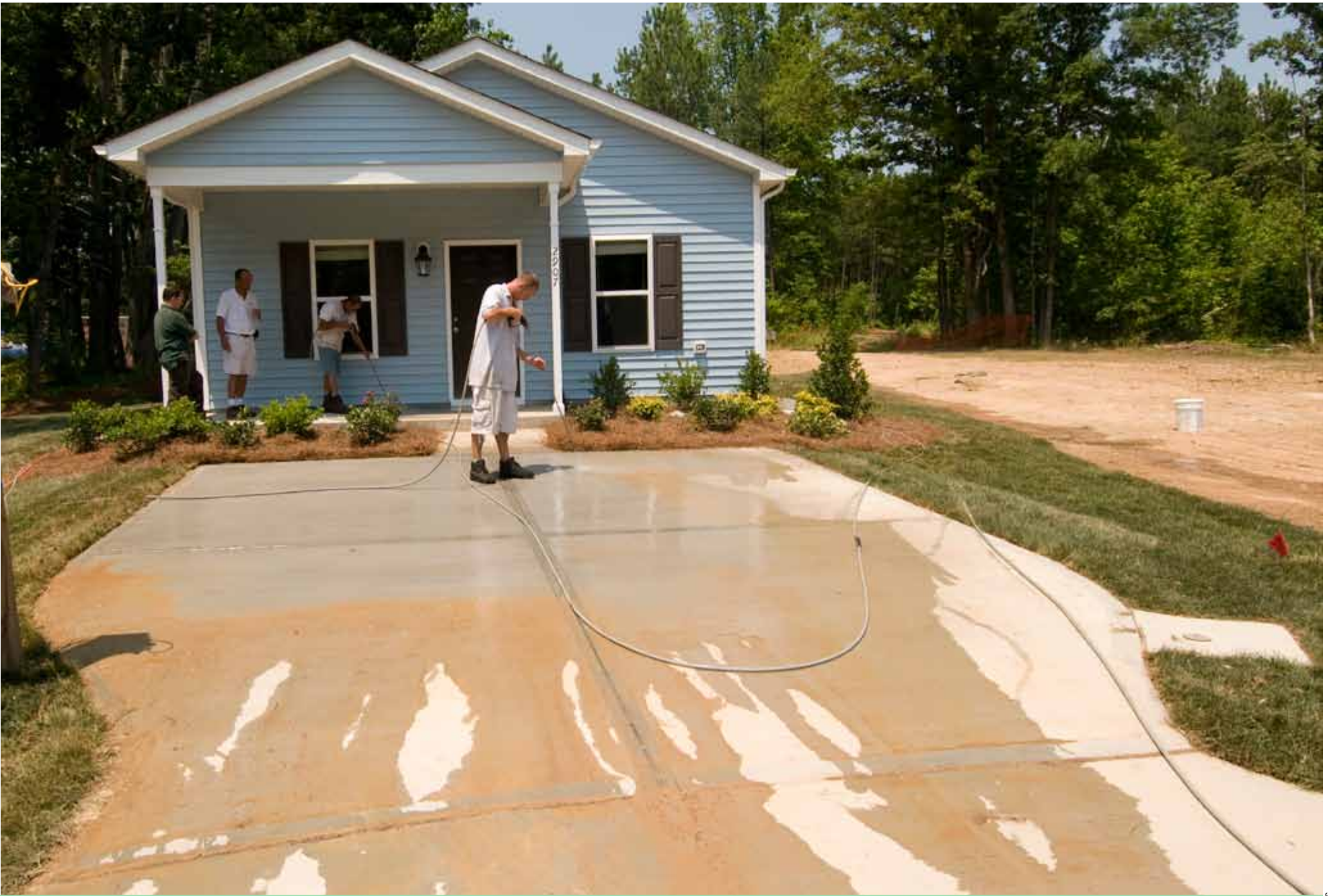
A power wash for the house and driveway helps get this Habitat house in Durham, N.C., ready for its owner.
