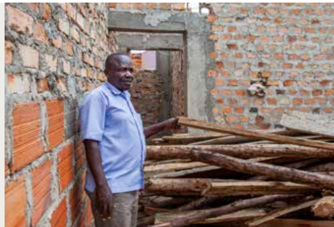
Wilfred observes the progress on the new apartment where he is going to live with his family.
