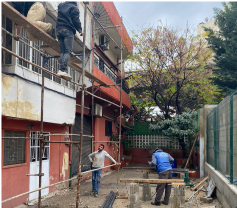
A multistory building's facade is repaired after damage caused by the Beirut Port explosion in Lebanon.
