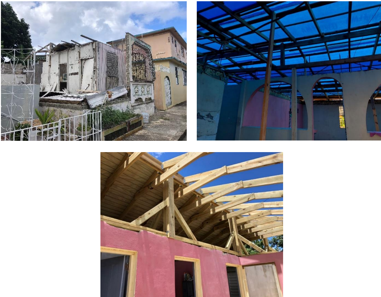
Figure 1. Houses in Puerto Rico in various states - abandonment (top left), temporary repairs (top right), reconstruction (bottom)
