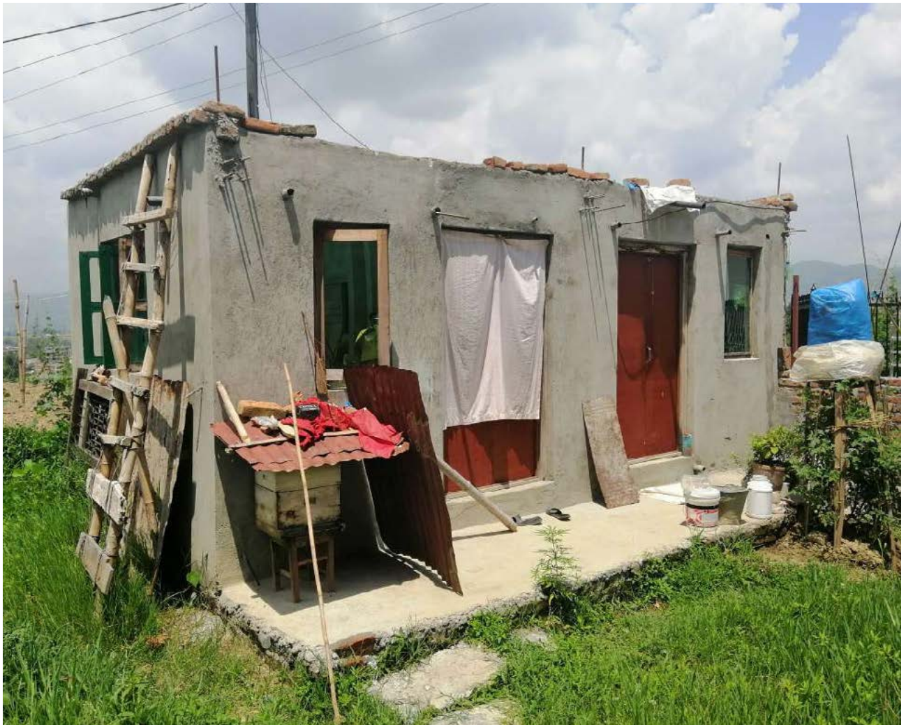
Single story two-room brick masonry house, incomplete and non-compliant, Suryabinayak. © Housing Recovery and Reconstruction Platform.
