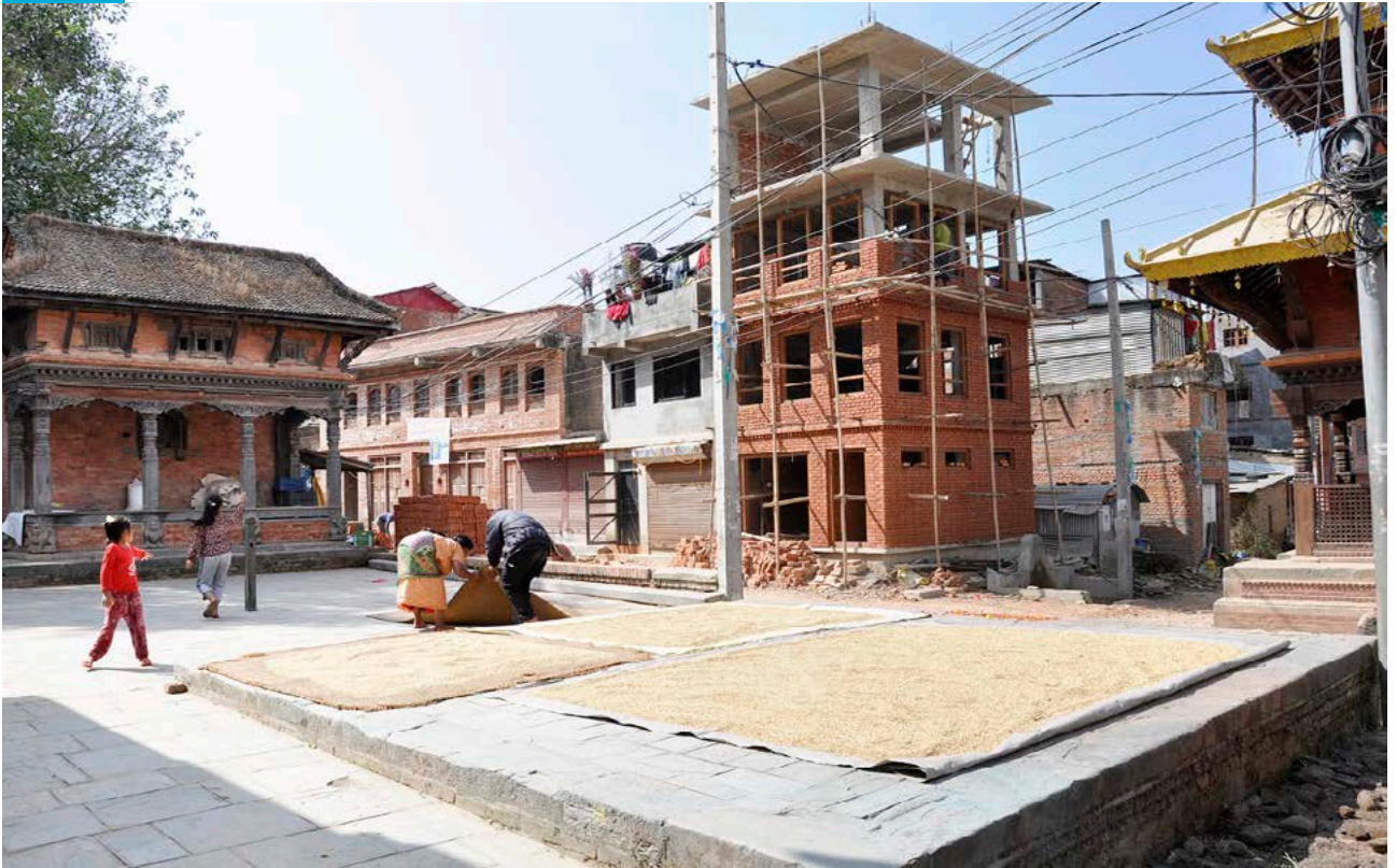
New construction, reinforced concrete frame but unrestrained brick walls. Municipal guidelines on materials and height applied.
