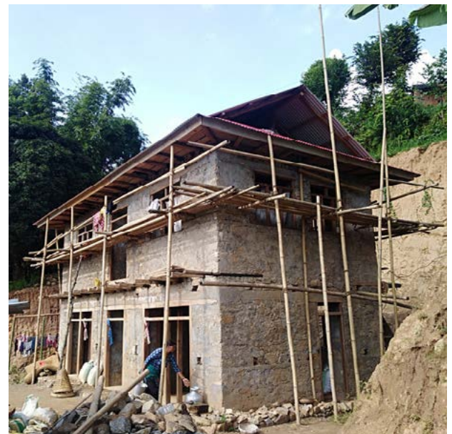
Stone masonry house Bhojpur municipality. House completed September 2018. © Housing Recovery and Reconstruction Platform.
