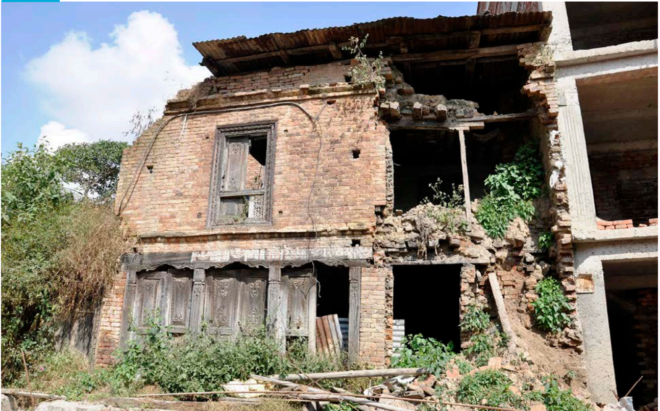
New building under construction adjoining damaged and abandoned building.
