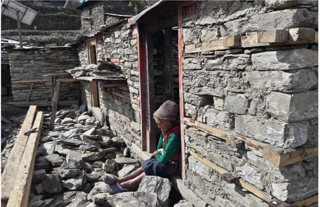
Rebuilding a home is particularly challenging for elderly residents. Sertung, Dhading, 2017. © Housing Recovery and Reconstruction Platform, National Society for Earthquake Technology, Nepal.
