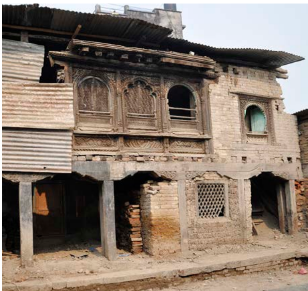
Damaged historic buildings one year after the earthquake, 2016.
