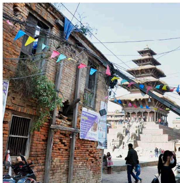
Earthquake-damaged unoccupied private house and shop propped for safety on busy public street, 2019, Bhaktapur.
