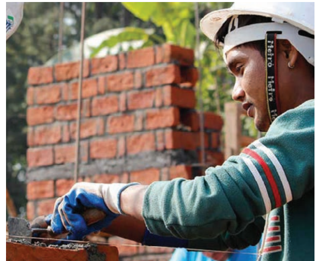
Quality assurance and basic skills are critical for safer reconstruction. © Habitat for Humanity Nepal.
