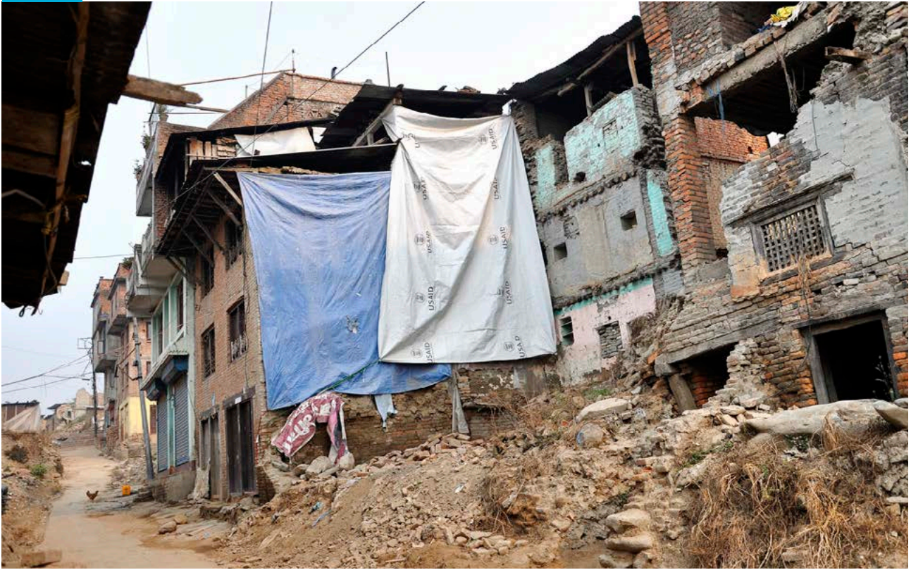
Damaged historic terraced buildings not weatherproofed or stabilized.
