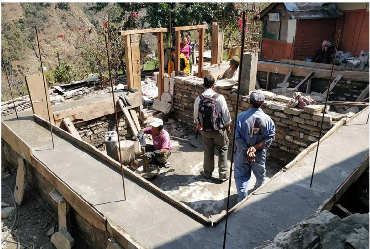
NRA engineers have unprecedented field knowledge of the housing sector from their recovery experience, Myagdi, March 2018. © Housing Recovery and Reconstruction Platform.
