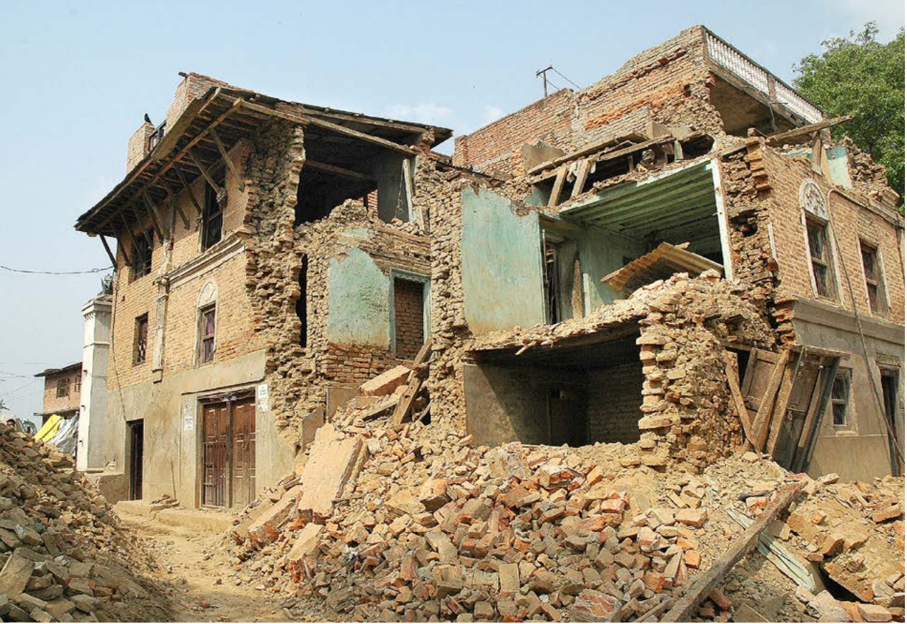
Bungamati damage to houses and workshops, 2015.
