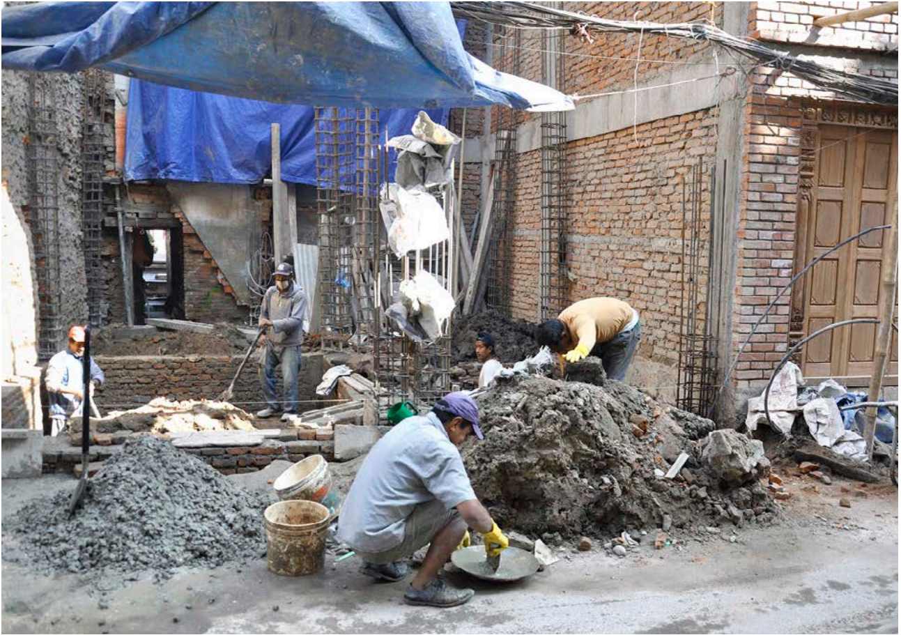
Reconstruction on small plot, storage of materials and preparation works on the main street Patan, February 2020.
