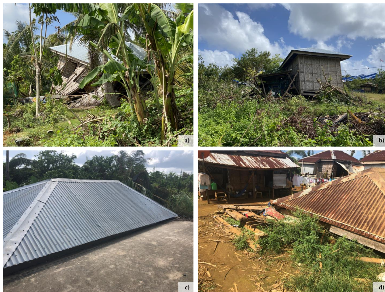
Figure 12: Examples of shelters that experienced wall failure due to failure of the column-foundation connection. a-b) Wall racking led to tilt and partial collapse. c-d) Wall racking led to complete collapse with roofs landing on the shelter. (Photos a & b by Abbie Liel).
