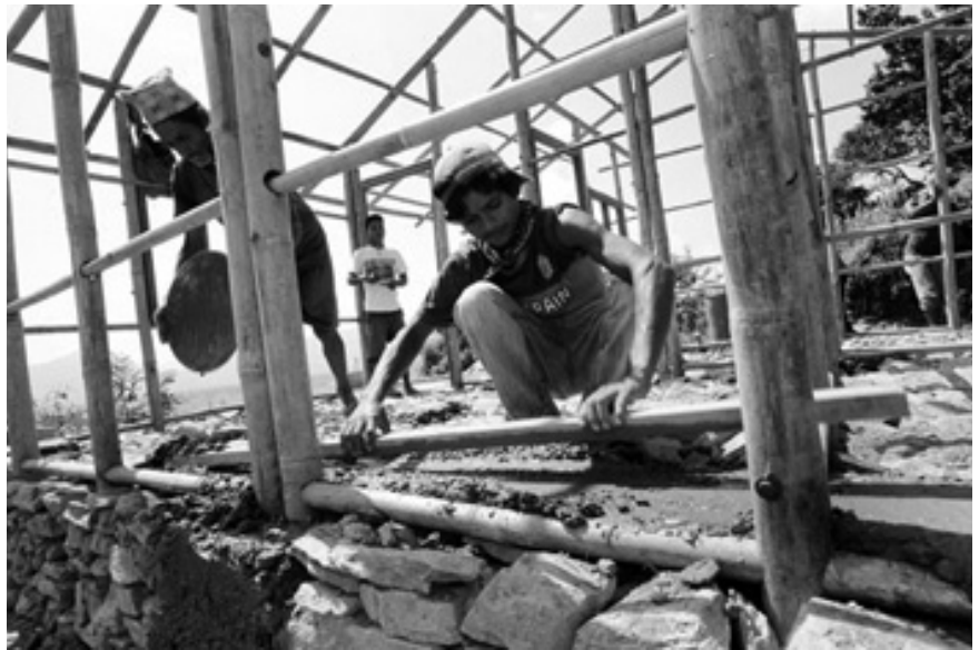
Putting to use cost-effective building technology based on local materials, home partners and local volunteers in Pokhara, Nepal, build frames of treated bamboo on a foundation of concrete and stone for the houses that were completed during Habitat’s Everest Build in October 2010. Home partners learn the bamboo construction techniques through a Habitat training program.
